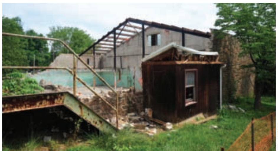
Photos of the NVF Corporate Headquarters before and during the demolition. This building, originally built as a rag warehouse in 1935, is the first phase of demolition and remediation of the floodplain along the Red Clay Creek.
